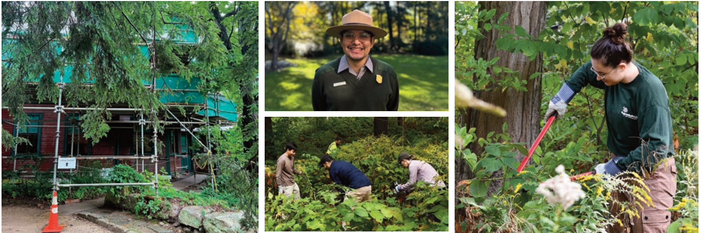
Left: Scaffolding on the historic building; Top center: NPS staff; Lower center and right: invasive species management. Courtesy NPS, Olmsted NHS.
